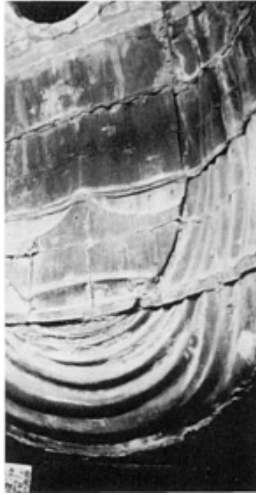
Fig. 13 View of the interior of the Kamakura Buddha showing the interlocking joints between the casts.
